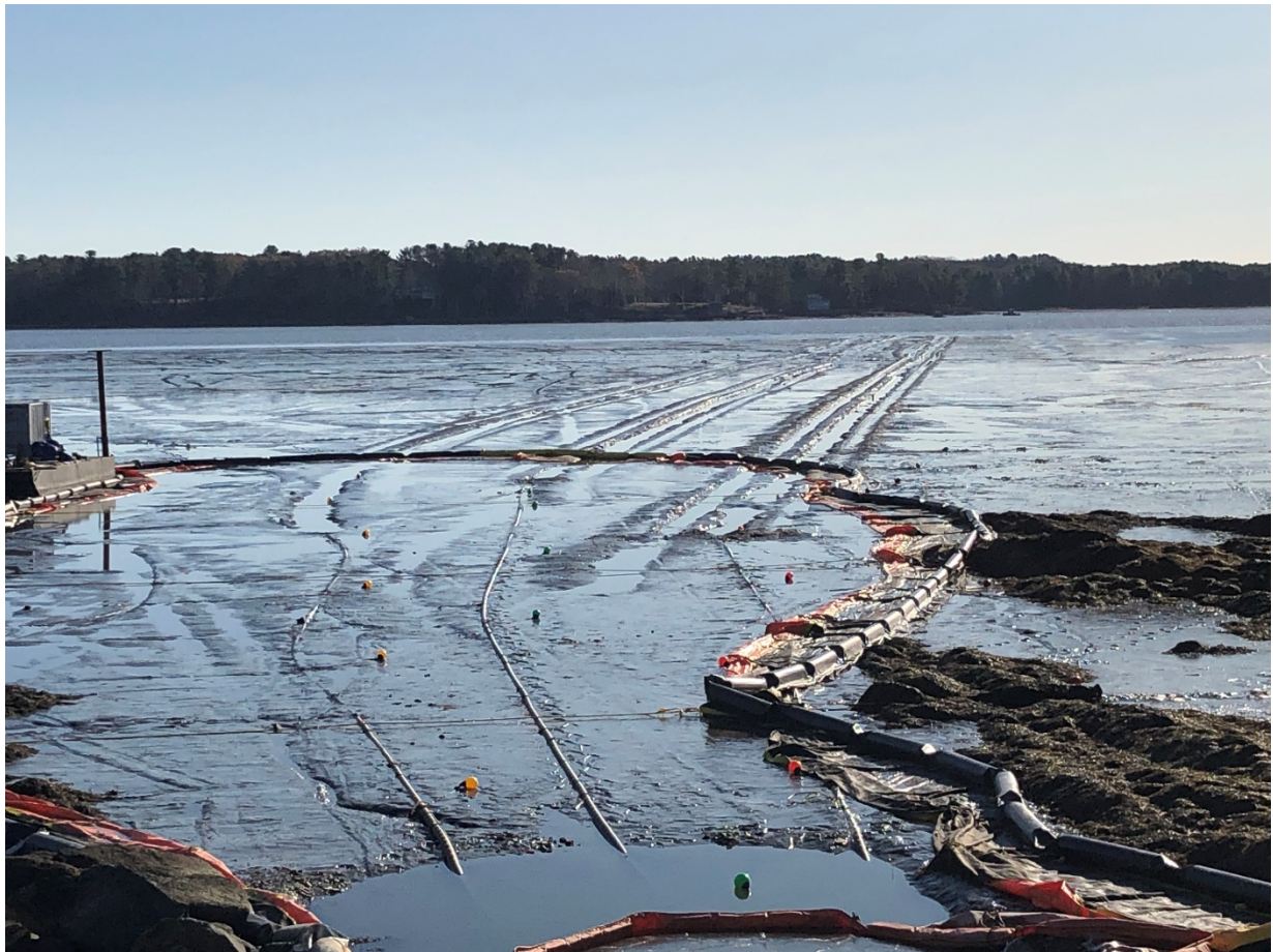
Photograph taking from Durham landfall location looking toward Newington landing along SRP submarine cable alignment during low tide (0845) the morning of 11-16-19 indicating bottom disturbance from jet plow installation of the three cables. Evidence of diver burial (hand-jetting) results on the northern cable inside of the turbidity barrier (left side of the photo closest to small spud barge).
